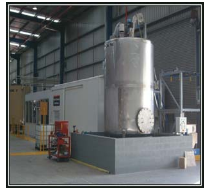
Fig 1. Cummins Filtration AdBlue ® Production facility in Melbourne
